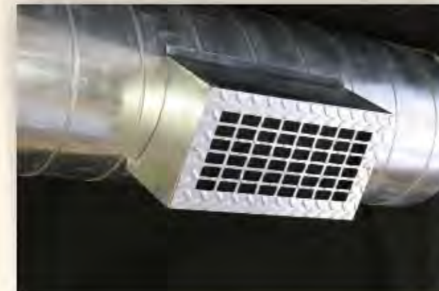
Spiral Duct in Sports Bar
