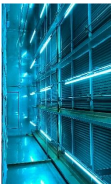
Air Handler Disinfection
